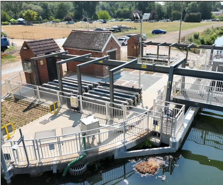
The entrance to the in-channel fish pass, with debris deflector plate, with eel pass discharge (green pipe).
