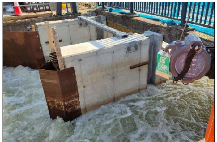
Steel protection to the new downstream sections of wall to reduce the potential for debris build-up on them over the winter
