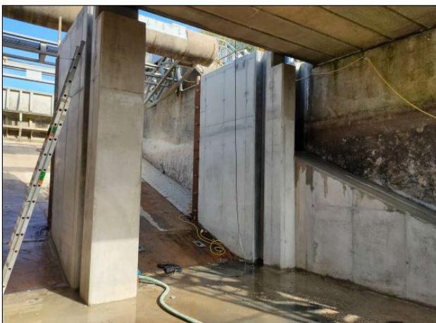
Parts of the new walls downstream of the existing gate including a section of the new fish pass
