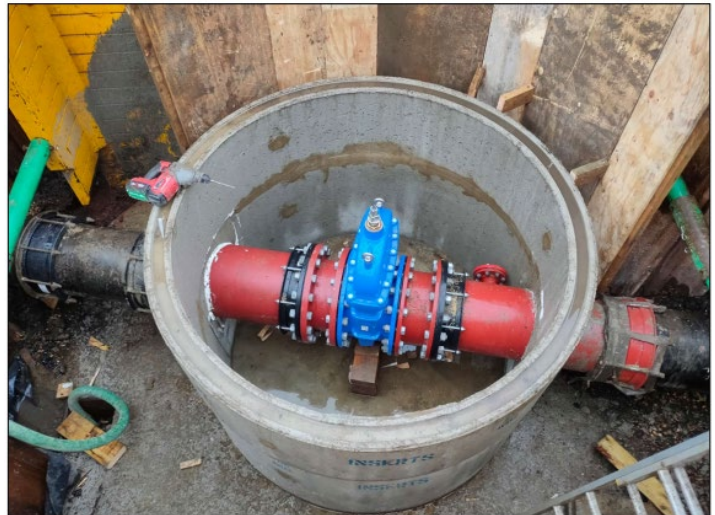
New valve and chamber in the bypass pipe to fine-tune very low summer flows
