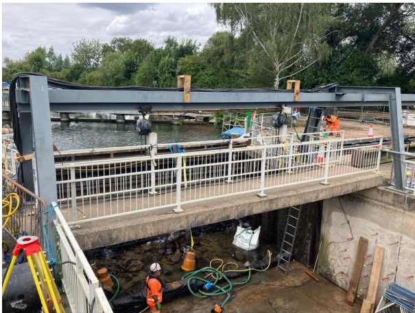
The stoplogs installed to isolate the sluice gate and water being pumped out to allow construction work to start.
