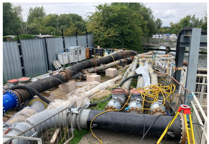
The temporary pump pipework to carry the summer river flows around Stanstead Sluice.
