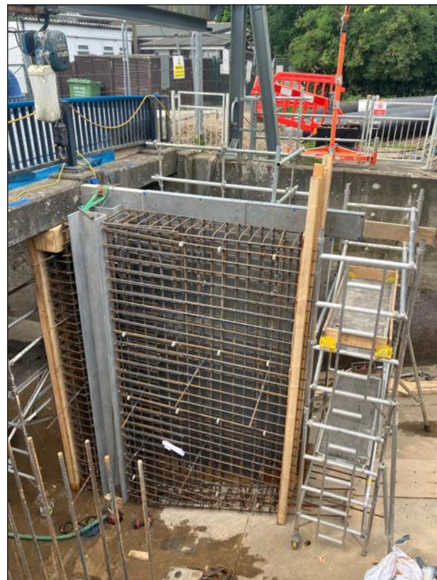
The reinforcing bars in place for the lower part of the wall that will divide the two new gates. It is ready for a final shutter to enclose it before concrete is poured around the reinforcing bars.
