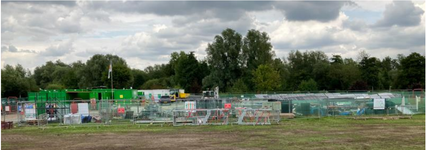
The construction compound near Stanstead Sluice with its temporary solar panel array.
